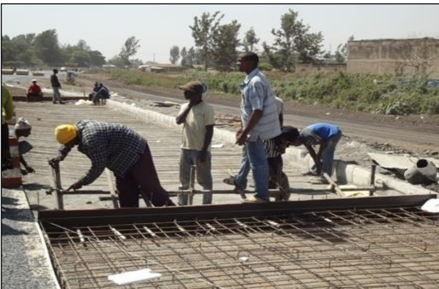
Figure 1: Chine Geo Construction Corporation workers working with no protective gear
