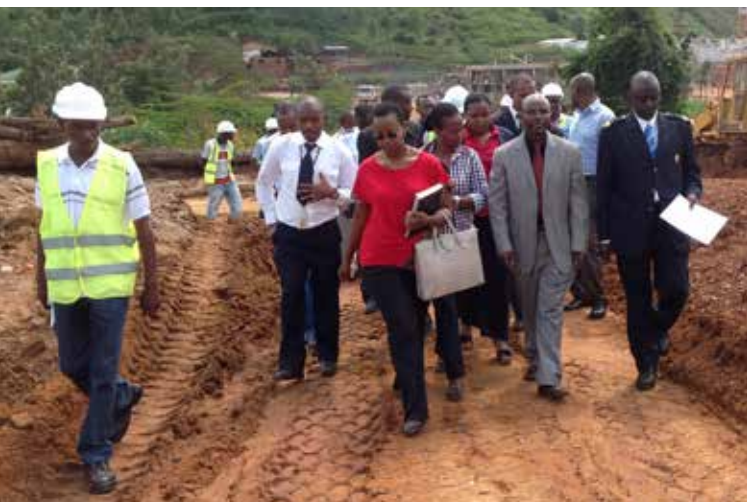
MINEAC's Permanent Secretary Mr. Innocent Safari (2 nd right) and stakeholders visiting the ongoing construction of Kagitumba OSBP - Mirama Hills.
