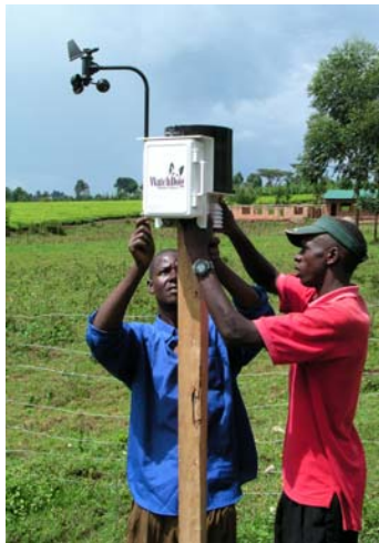
Figure 5.17: Watchdog Weather Station Installation at the Township Primary School
